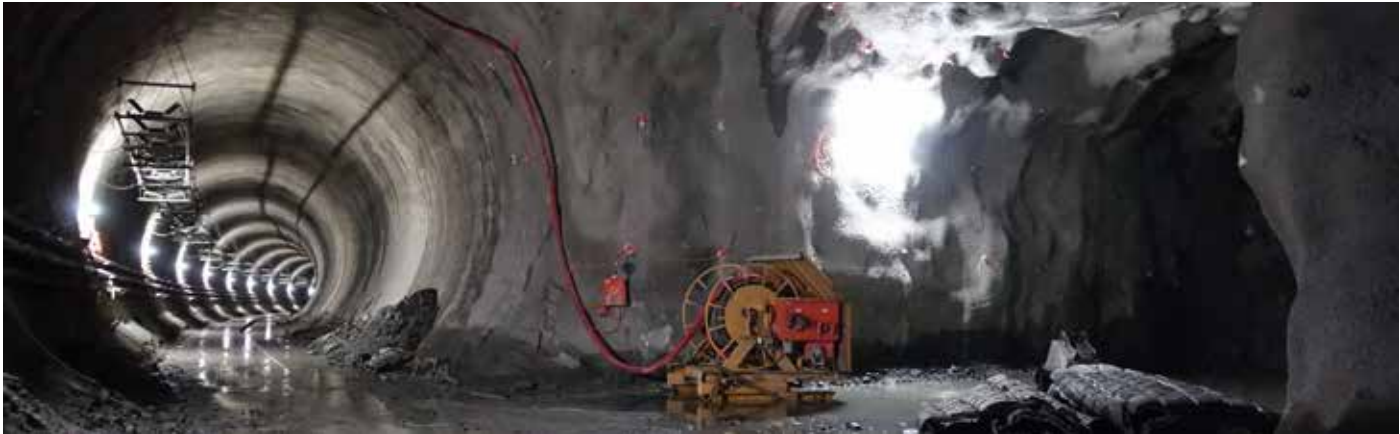
One of the 16 cross passages between the new and the original Ulriken tunnel (to the right). Left: New Ulriken tunnel. Photo: Ingvild Eikeland, Bane NOR
