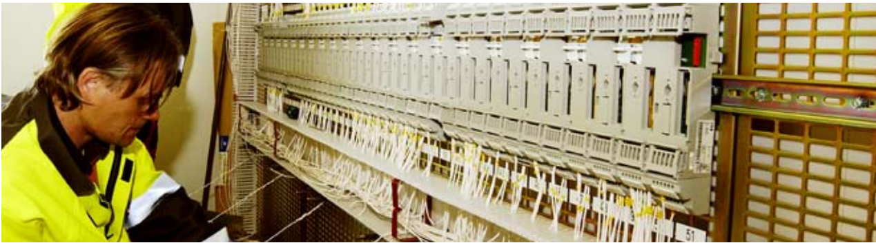
Part of safety installation. Photo: Jernbaneverket
